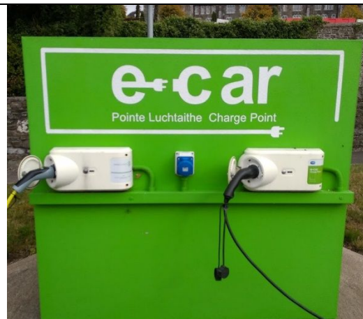
Example of Charging points for EV (University College Cork, Ireland)
